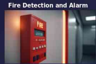
Fire Detection and Alarm
